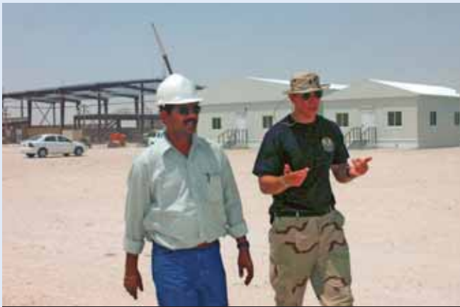
First Lieutenant Steven Thomas (right) works closely with local contractors on construction projects at Al Udeid Air Base, Qatar.
