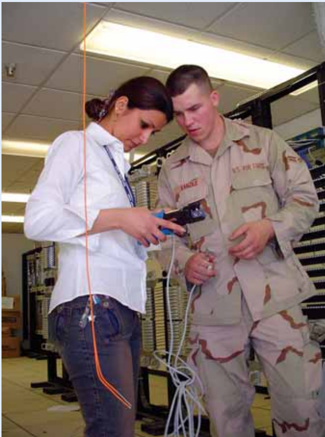
In Baghdad, Iraq, Contractor Sarah Izet and Airman 1st Class Brandon Vanzile attach connectors to communications wires to help bring high-speed access to the Baghdad International Airport.
